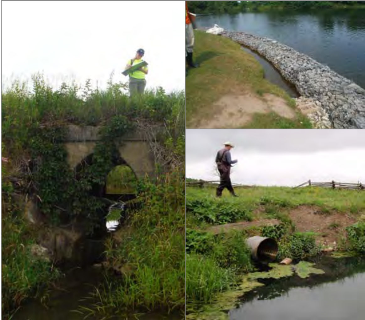
Figure 6-7: Examples of a weir, a failed bank hardening, and a perched culvert in the Whites Creek and Talbot River subwatersheds.
