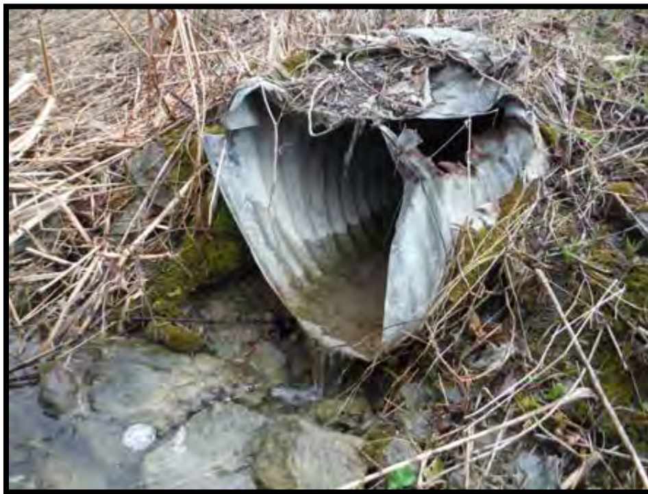
Figure 4-11: An example of a perched culvert on Georgina Island
