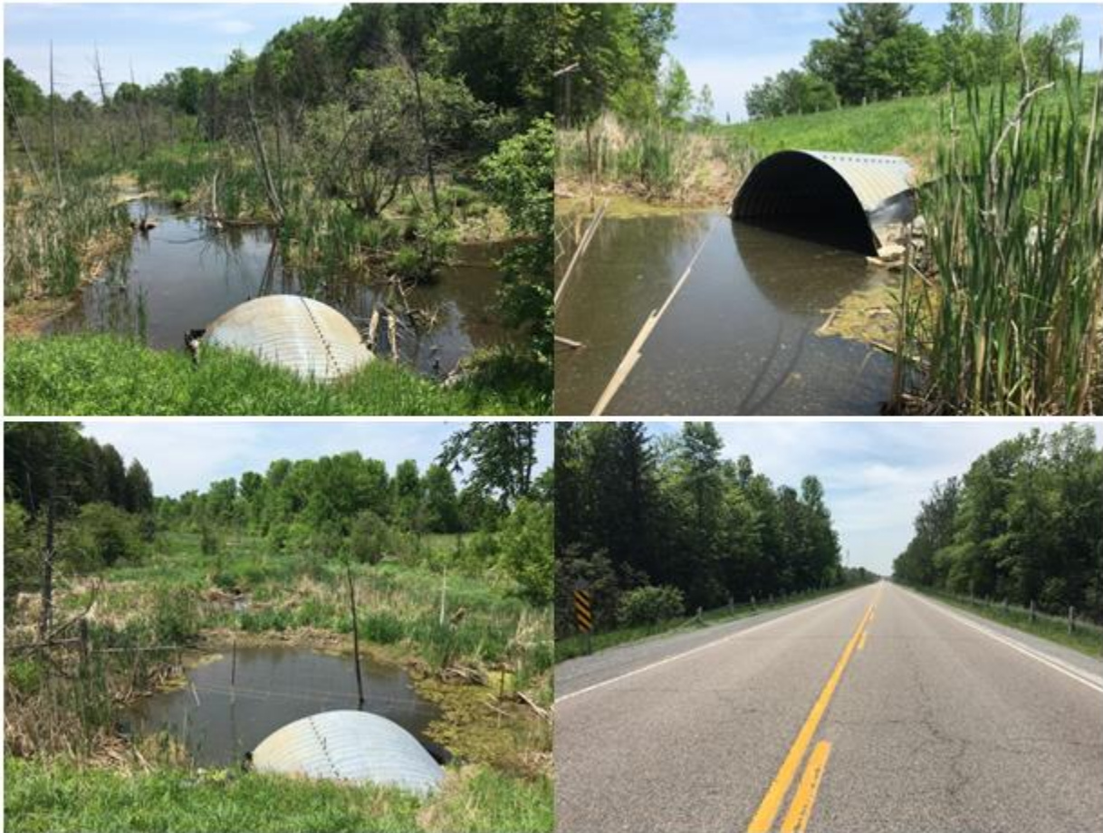
Figure 4. Photos of Site 3, clockwise from top left: view of culvert and wetland south of site; culvert, looking northwest; culvert and wetland on north side; view of road, looking west
