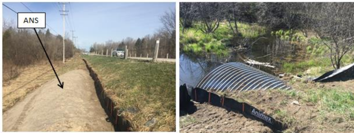
Figure 6. Ecopassage fence installation showing the below-grade design and artificial nesting structure (left), and the connection to existing road crossing infrastructure (right).
