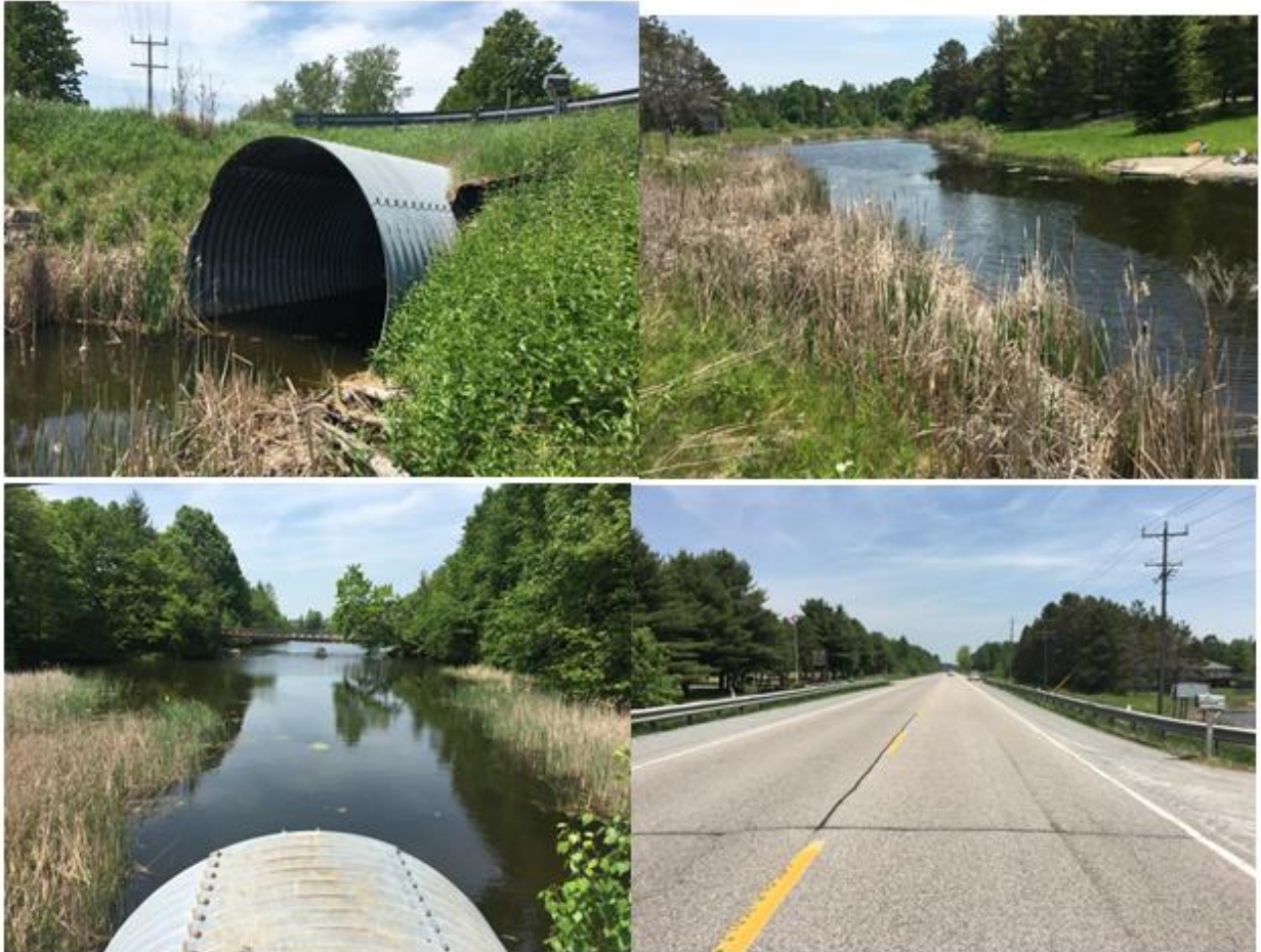
Figure 5. Photos of Site 4, clockwise from top left: view of culvert, looking northwest; open water and cultural thicket, looking southeast; open water (Talbot River), looking north; view of road, looking east
