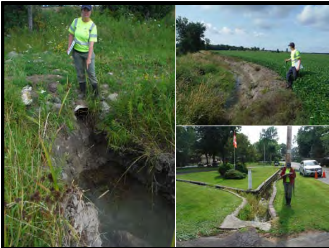
Figure 5-8: Examples of perched culverts, channelization, bank hardening, and barriers in the Ramara Creeks subwatershed.
