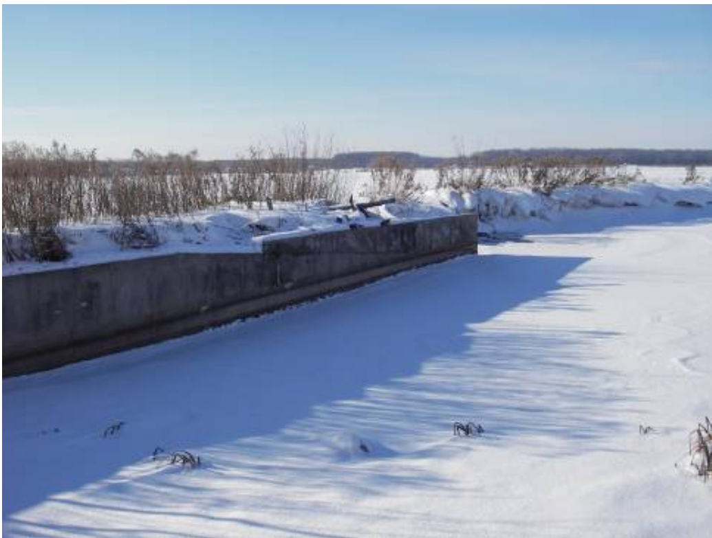
Figure 7-6 Channel hardening (Reach WH 18)
