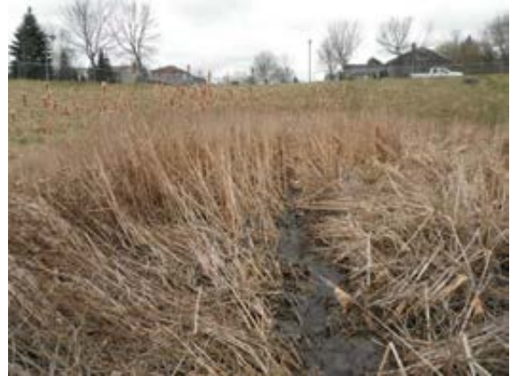
Figure 5 -Prior to the retrofit the facility consisted primarily of a grassed waterway
