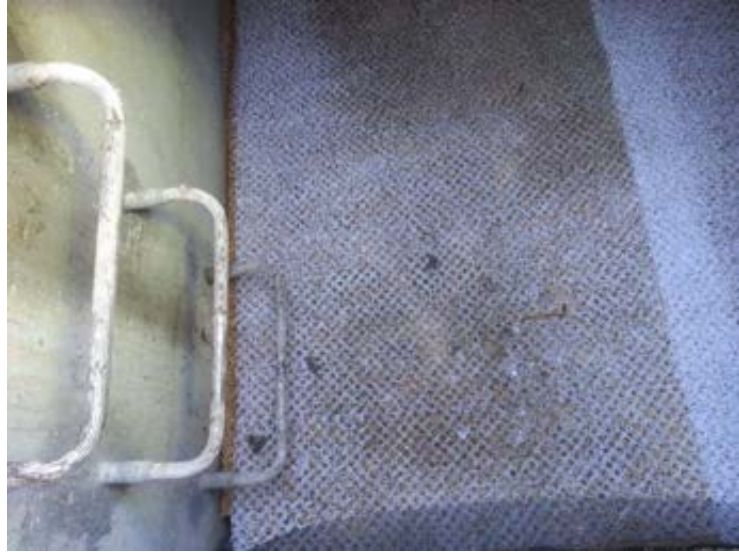
Figure 8 - View inside Sorbtive media chamber, media overlain with permeable layer to hold the Sorbtive media in place
