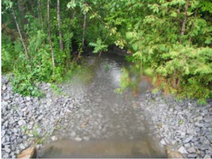
Figure 13 - Lincoln and King St outlet under high flow conditions. Water depth exceeding 20 cm.
