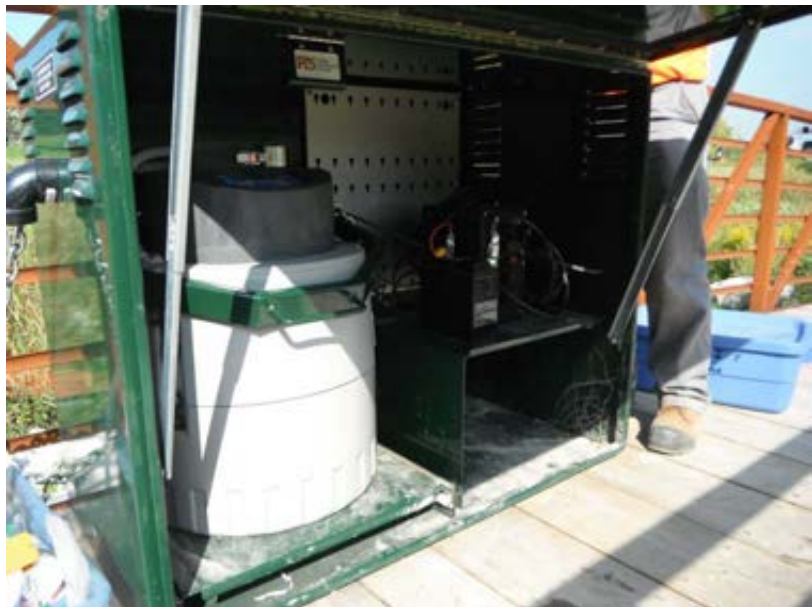
Figure 1 - Monitoring equipment setup at Colony Trail facility
