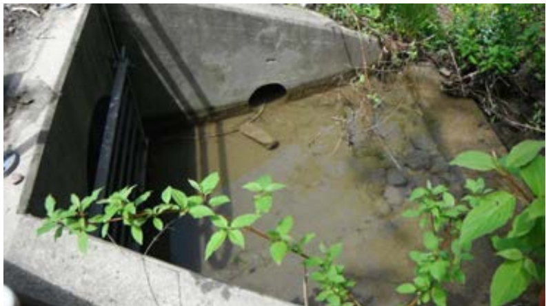
Figure 12 - Joint outlet of King St stormsewer and Lincoln facility under low flow conditions. Lincoln outlet is the small diameter pipe on right wing wall
