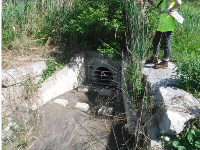
Figure 9: Sediment build-up/siltation in inlet of stormwater pond
