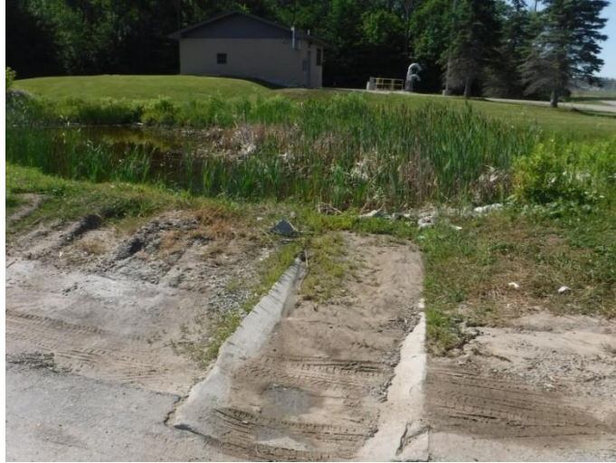
Figure 7: An inlet experiencing erosion/runoff from adjacent parking lot
