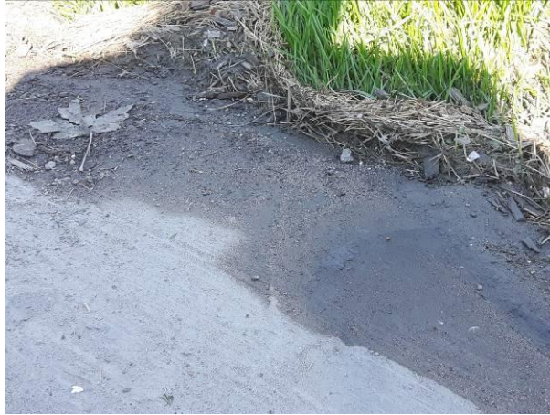
Figure 15: A bioswale with sediment build up/siltation
