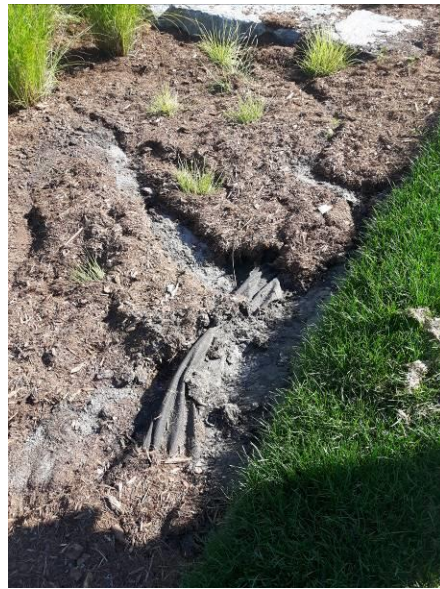
Figure 14: A bioswale with exposed bio filter and significant erosion of the top soil layer
