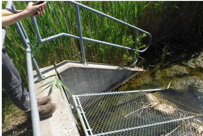
Figure 10: Debris in inlet obstructing flow
