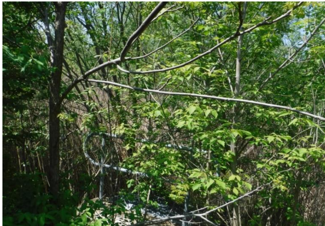
Figure 8: An outlet in heavily vegetated, not well maintained area
