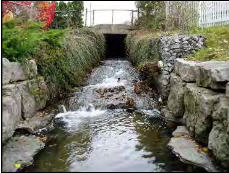
Figure 5-10: Example of barrier, bank hardening, and channelization on Kidd's Creek downstream of Thompson St, Barrie.
