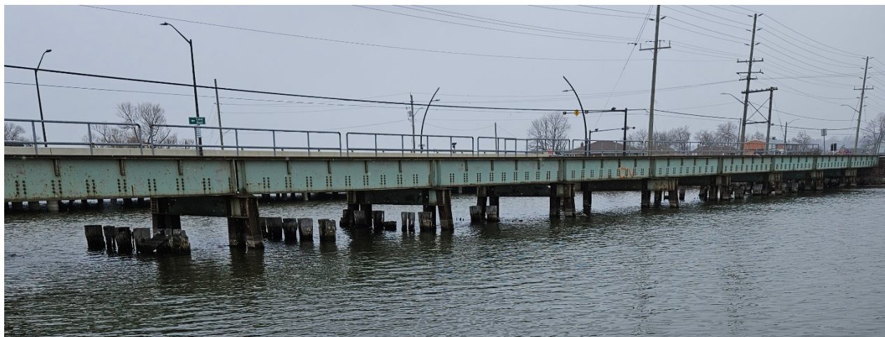
Figure 2. Wooden supports visible beside site TS-7, where elevated concentrations of PAHs were detected.
